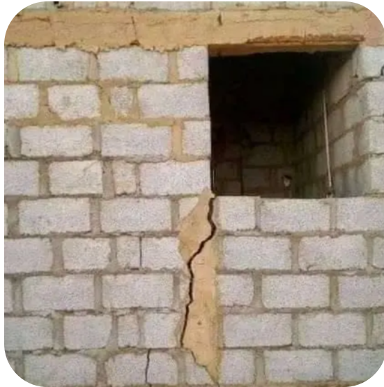
Cracks in wall
