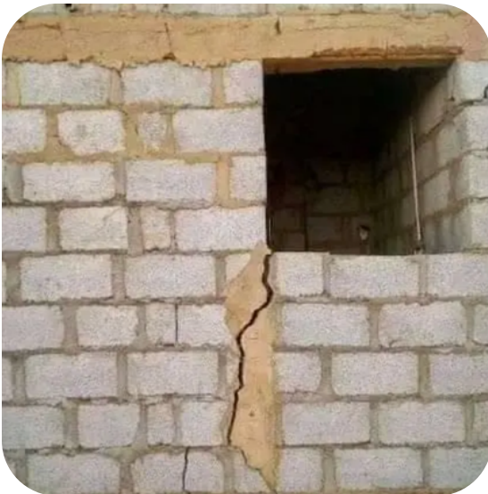
Cracks in wall
